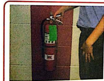
A If a fire breaks out in your shop, quickly walk to the closest fire extinguisher and lift it off of the wall.
